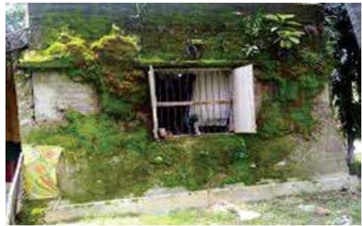
moss on the wall
